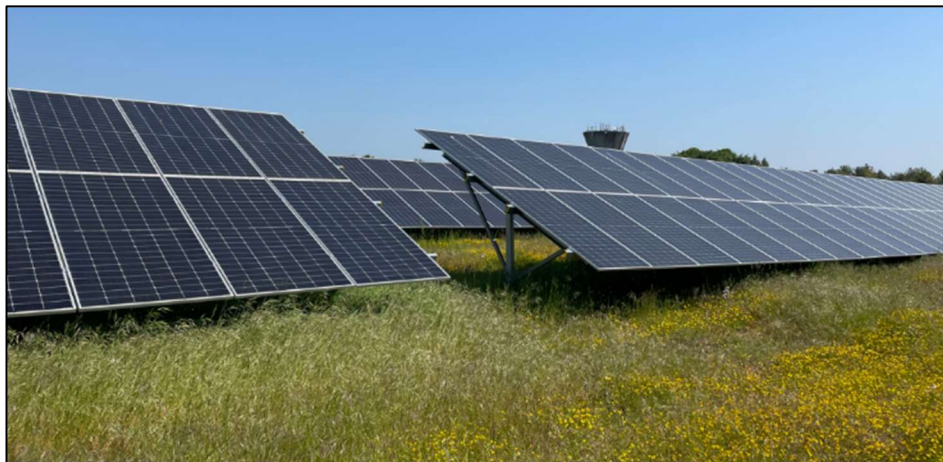
Figure 8.3: Example Side view of PV Arrays
